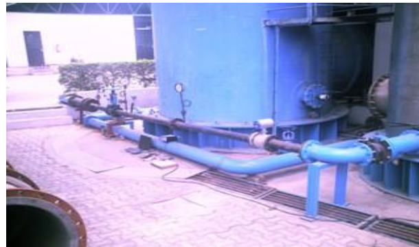
Figure 4. Test Rig for control valve
