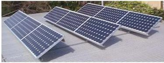
FIG: VIEW OF SOLAR CELL PANEL
