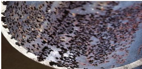
Fig: 2 Oxygen pitting of a boiler feed water pipe.
